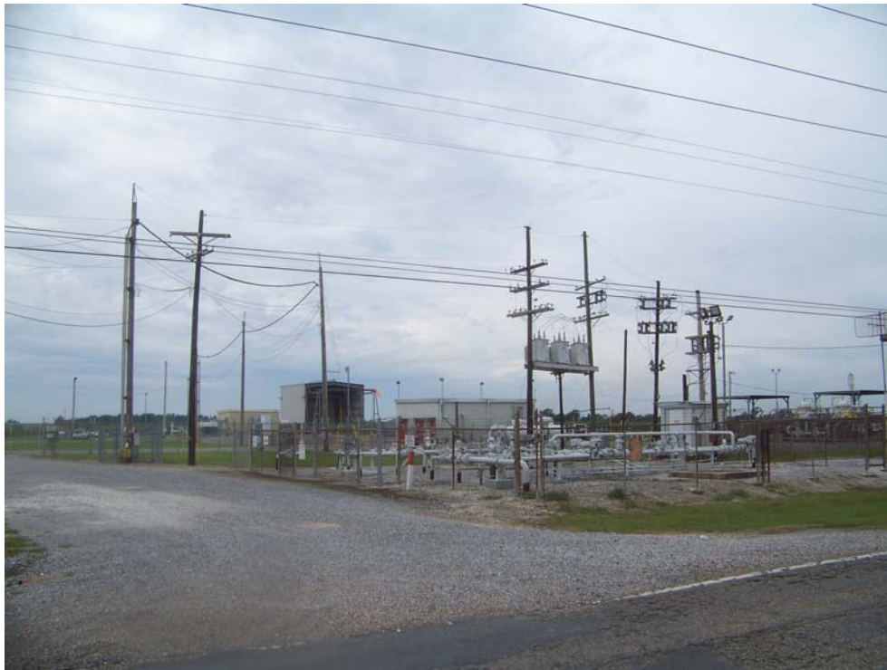
Photograph 16. Adjacent pipeline gathering facility
