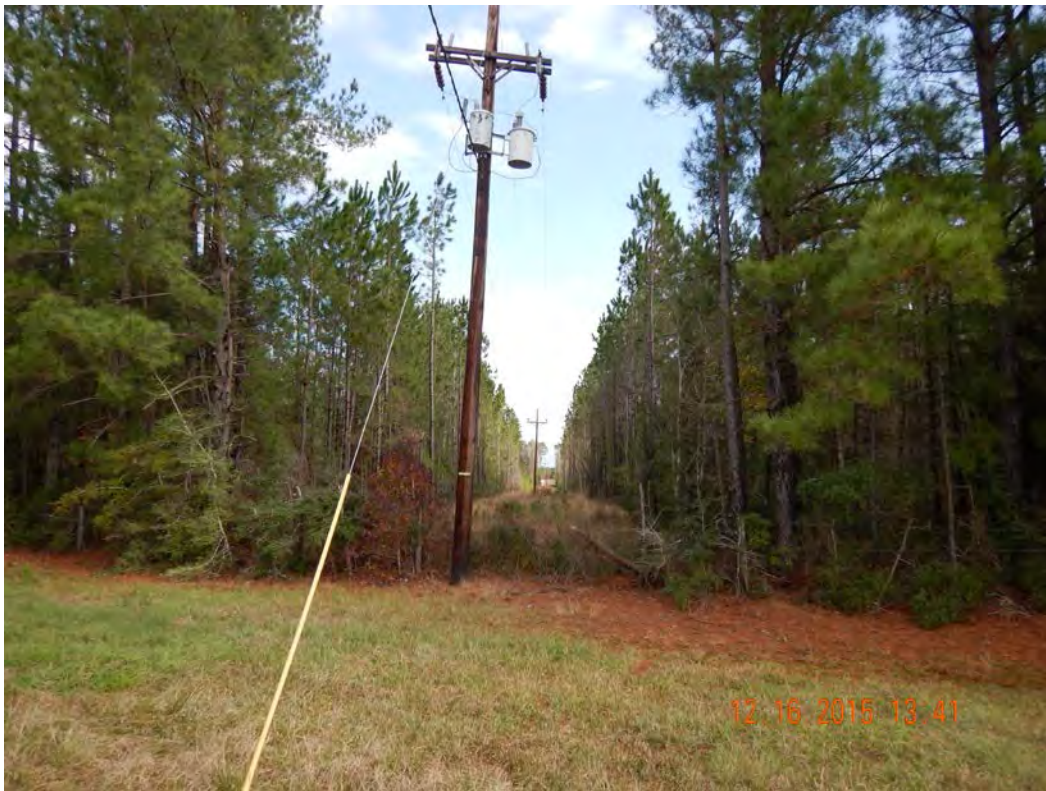
Photograph 14. View of power lines with transformers at orchard buildings; from west to east.
