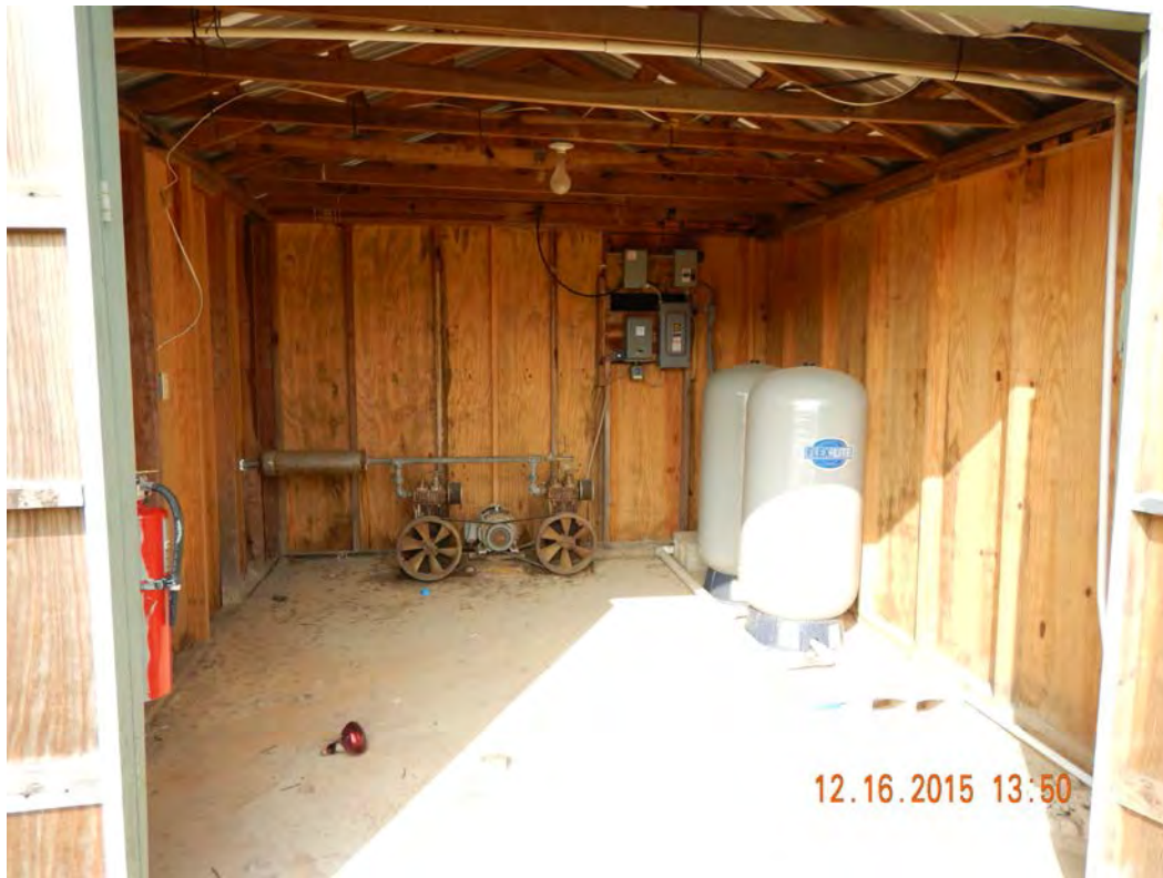
Photograph 23. Orchard irrigation well pump house interior with pump motors and two fiberglass treatment tanks.
