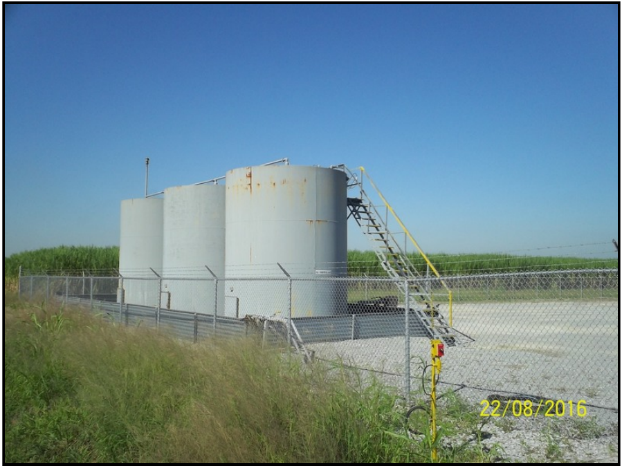
Photo 7: Appearance of three (3) ASTs in connection with gas production facility located on south adjoining property.
