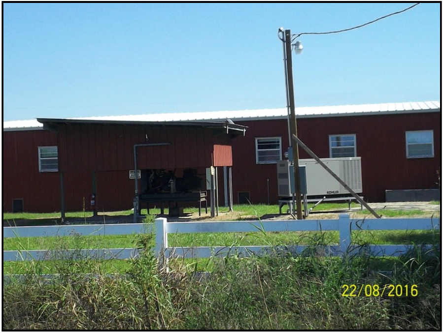
Photo 47: View of generators on the Maintenance Enterprises site from the subject property.
