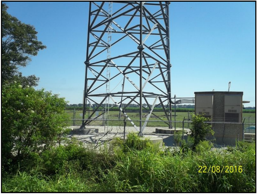
Photo 41: View of the base of the cellular tower and compound located on the northeast adjoining property.
