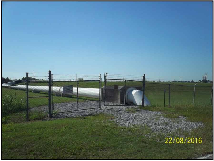
Photo 3: View of waste water pipeline into the Clean Harbors waste facility off Clark Road facing south.
