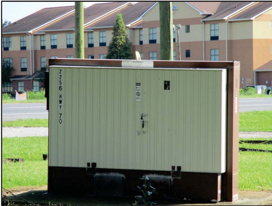
Photo 6: Appearance of a pad-mounted transformer located on the adjoining property to the northeast.
