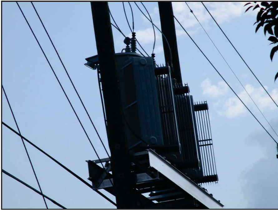
Photo 5: Appearance of three transformers on the adjoining property to the northeast.
