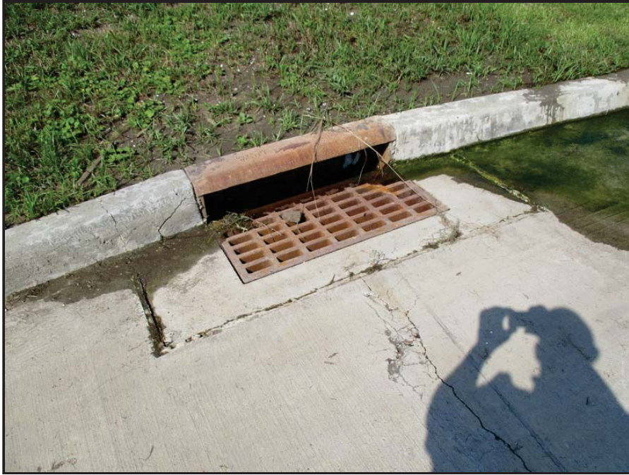
Photo 33: Appearance of a stormwater drain located on the Tractor Supply drive.
