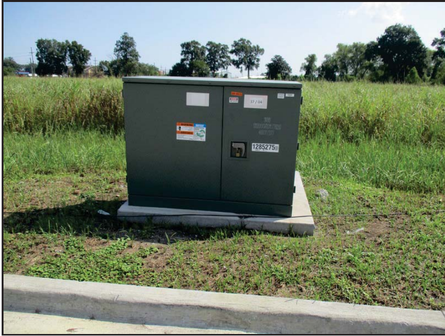
Photo 35: Appearance of a pad-mounted transformer located on the adjoining property to the west of the subject property.
