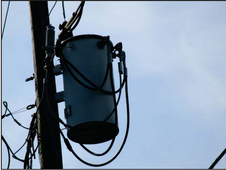
Photo 7: Appearance of a pole-mounted transformer located along the eastern section of the subject property.
