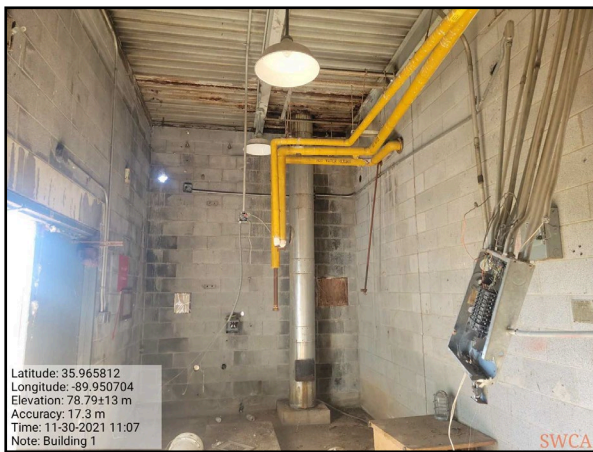
Photo 5: Interior of electrical room in building #1.
