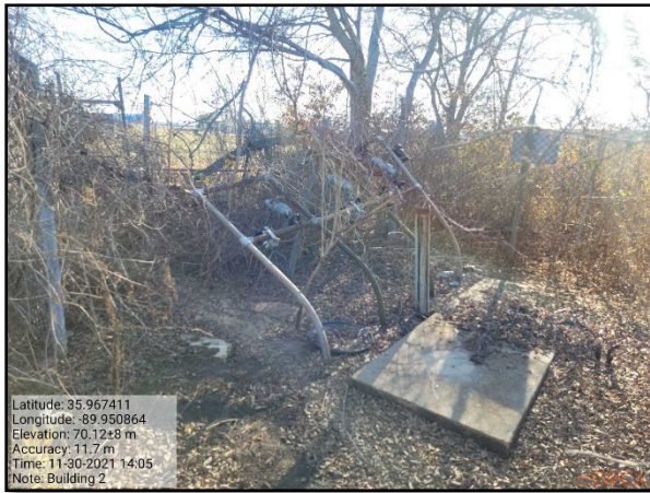
Photo 11: Dilapidated electrical controls stand outside of building #2.
