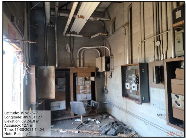
Photo 10: Interior of electrical room in building #2.
