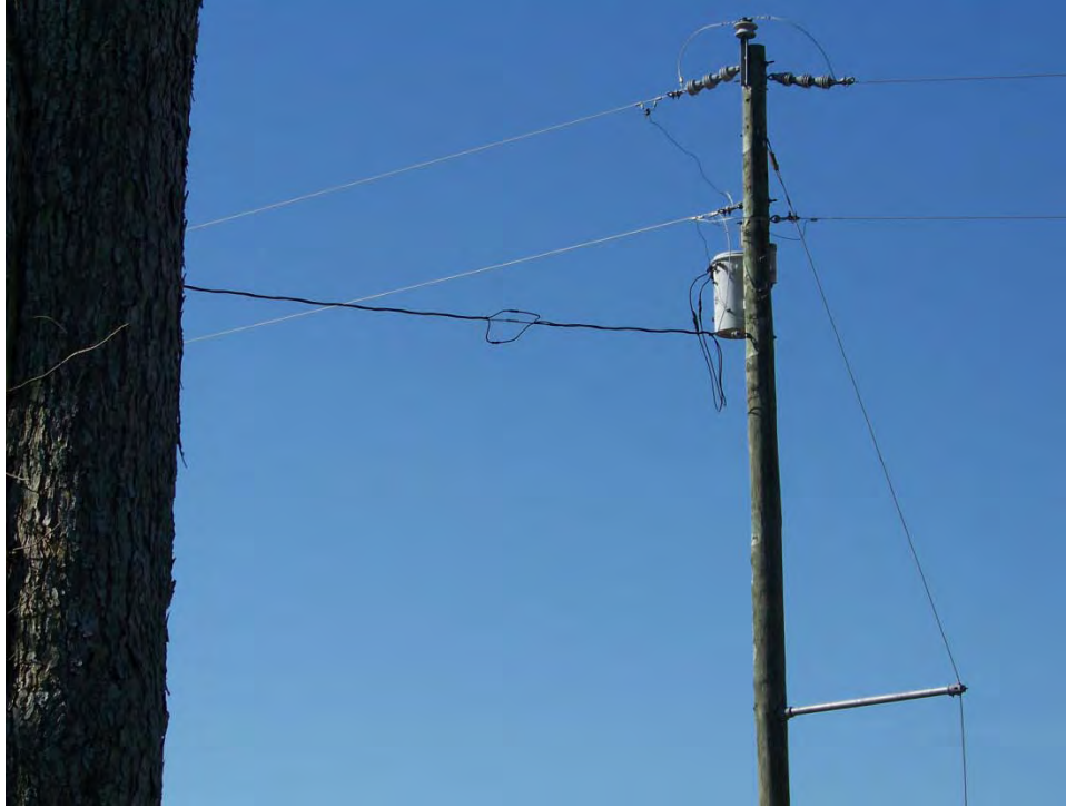
Photograph 7. One of two pole-mounted transformers on eastern edge of property near LA 3000/76
