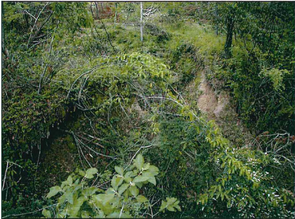
Figure 8. Photograph illustrating erosion of steep slopes in western portion of the proposed power generation facility.
