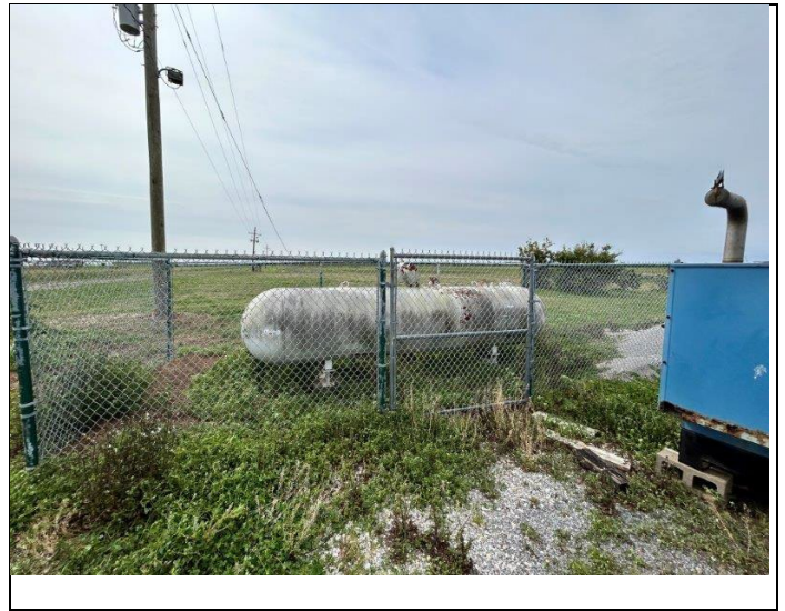
12. Propane tank associated with Natural Resources Conservation buildings
