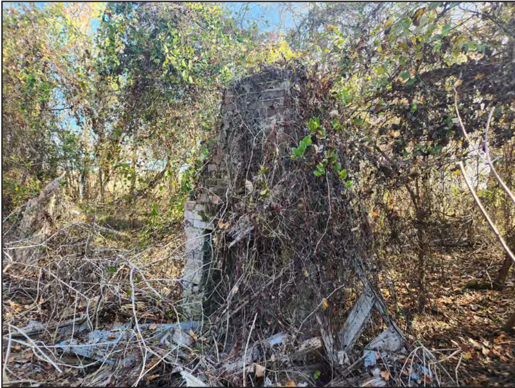
Figure 5.21. View of the standing chimney base surrounded by the collapsed structure, facing east-northeast.
