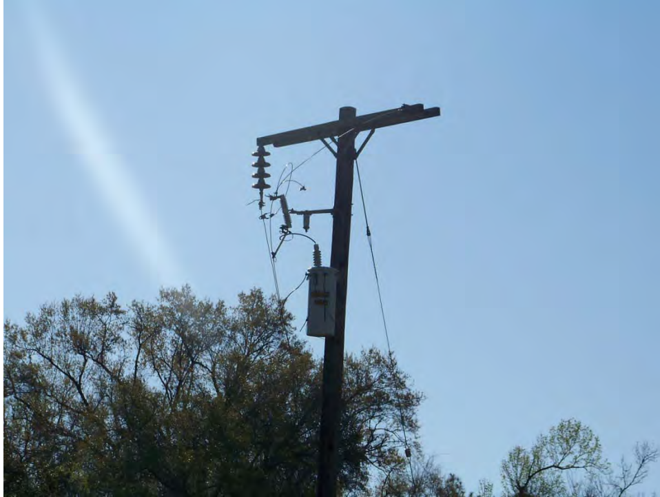
Photograph 7. One pole-mounted transformer on southeastern edge of property
