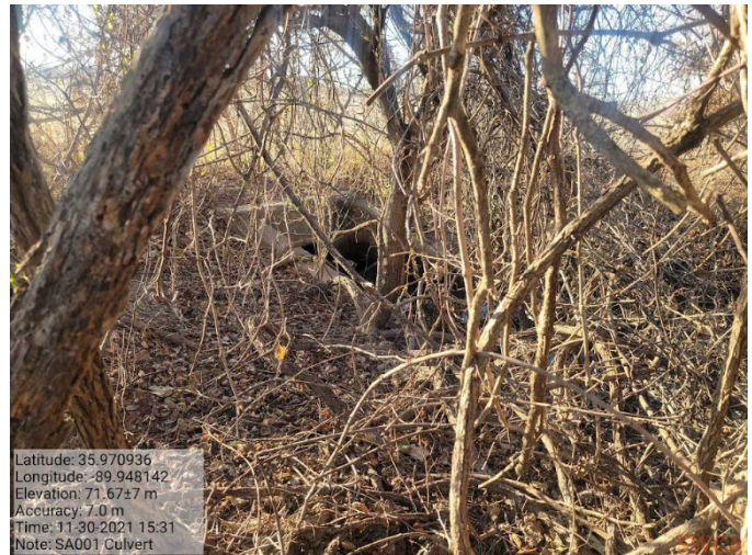
Photo C-4. Discharge culvert located within agricultural field drainage WCA001 and overgrown woody vegetation.
