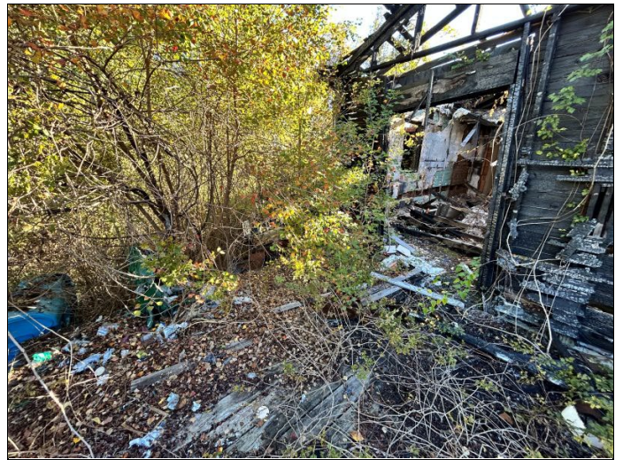
34. Fire-damaged house in eastern part of the property
