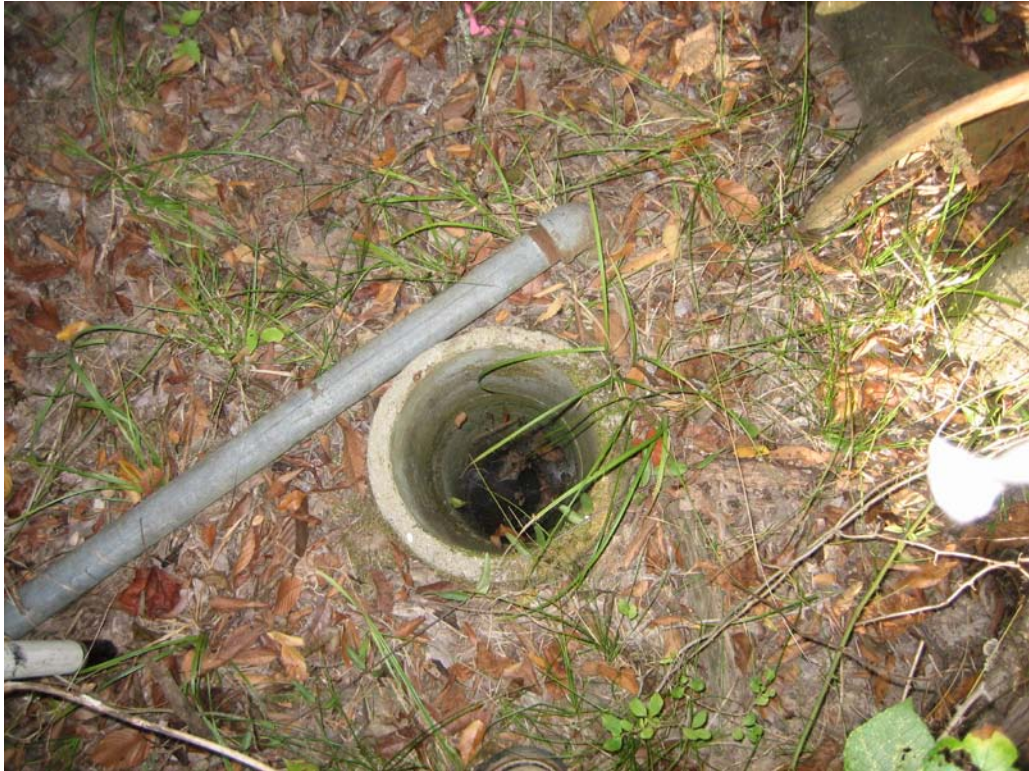
Open water well located near the northeast corner of the assessment property.
