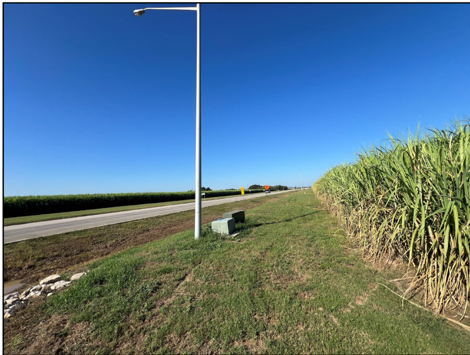
Photograph #4. SE corner of Subject property looking east, pad-mounted transformers visible.
