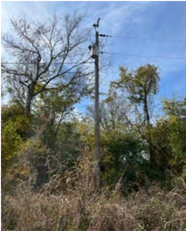
Transformer 2 on east side
