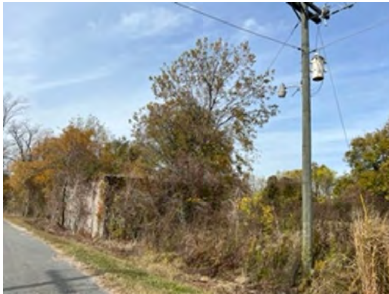
N. End looking north with transformer 3
