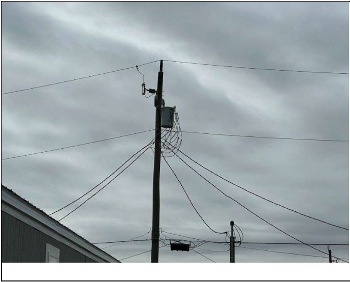
13. Transformer (3 pole mounted) associated with trailer
