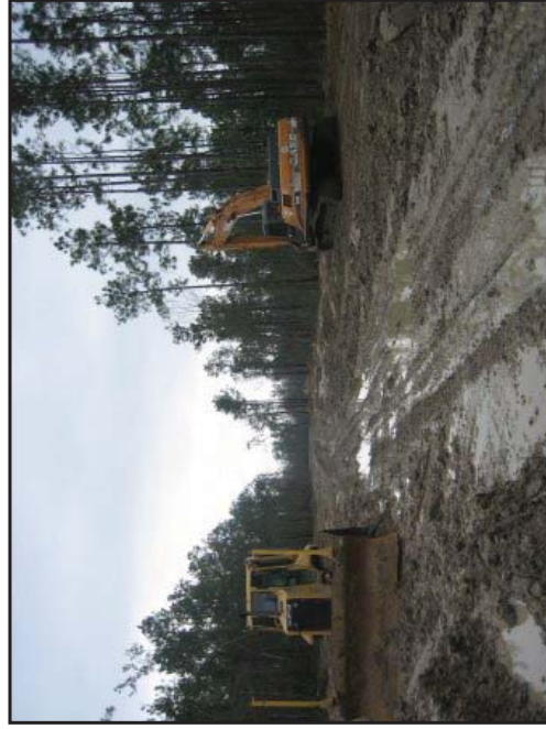
View of the remaining construction corridor for Summit Boulevard and general construction equipment facing south.
