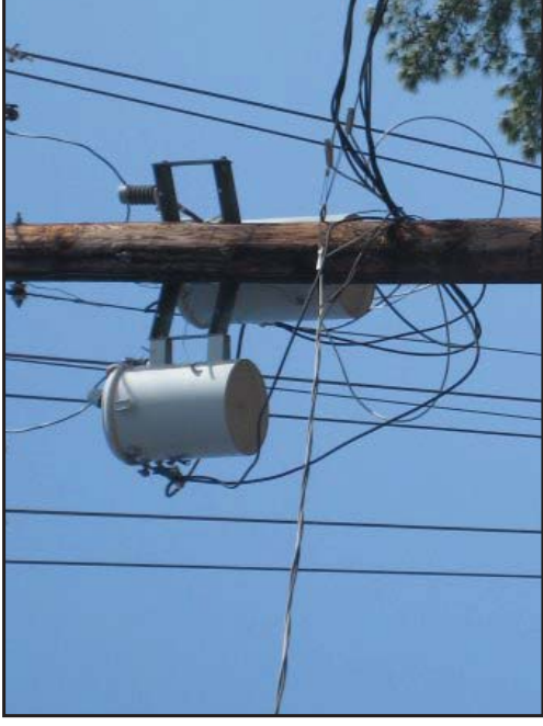
Representative view of the transformers located on Daney Street along the northern boundary of the subject property.
