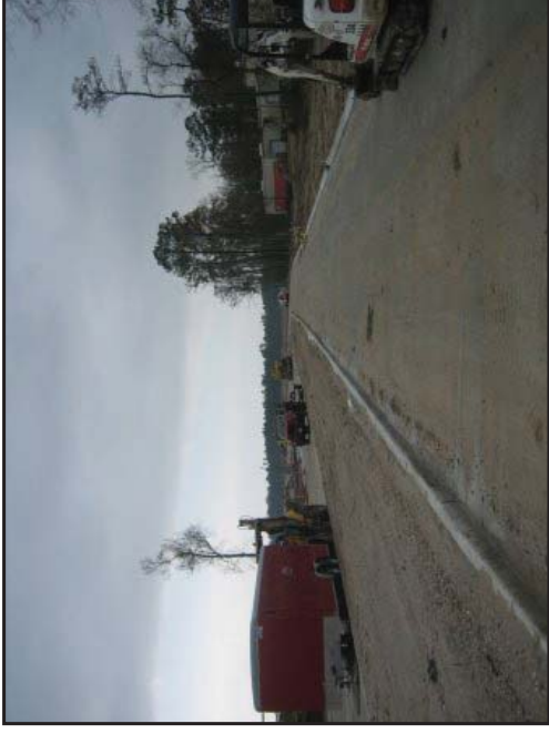
View of new construction of Summit Boulevard at intersection with Highway 190 facing south.
