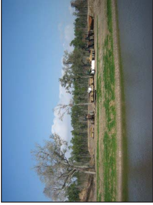
View of the w-14 Canal and construction equipment, including ASTs, on the southern portion of the subject property facing north.
