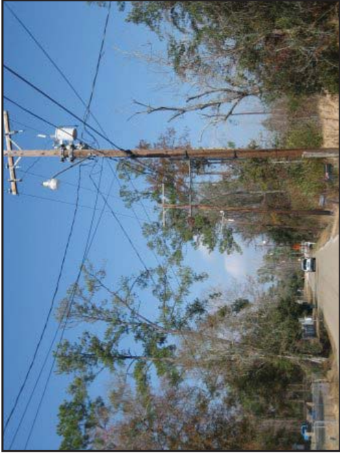
View of transformers along Nellie Drive, north adjoining property to the subject property, facing north.
